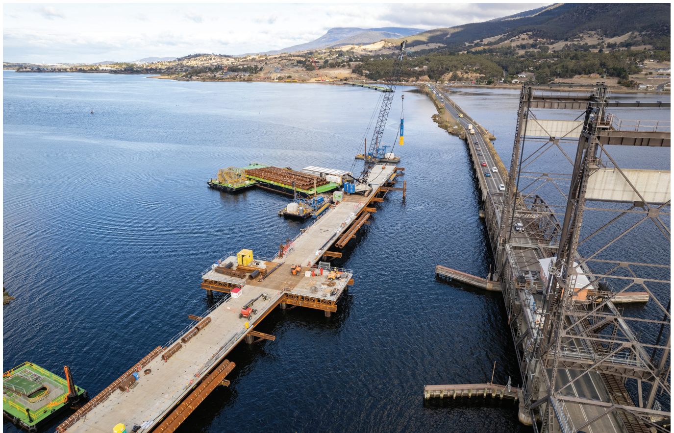
Construction of the temporary bridge continues to progress, with the remaining six barges being installed.
